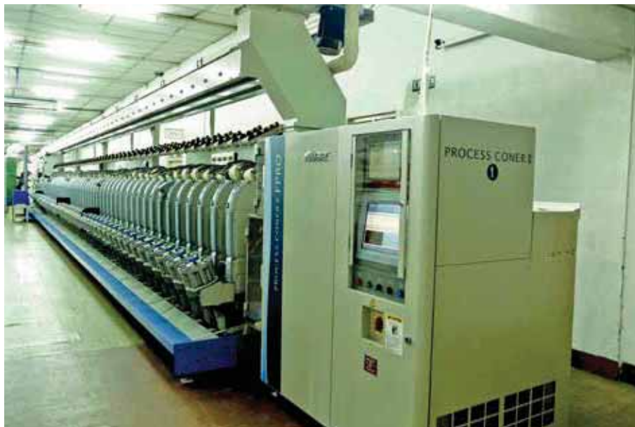
New “Murata FPRO Drumless” Auto Cone Winding Machine installed at our unit Rajapalayam Spintex, Rajapalayam.
